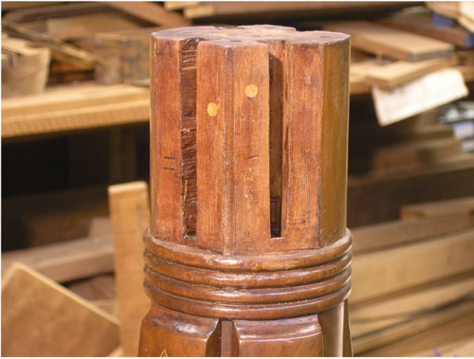
Fig. 8. Another view of the pedestal column with the dowels from a previous repair.
