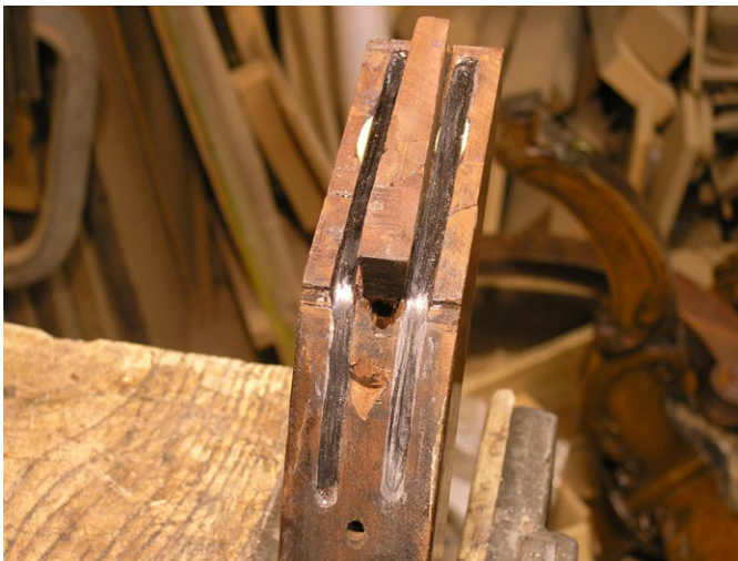
Fig. 6. Reinforcing the leg with strips of carbon fiber-reinforced epoxy in shallow grooves.
